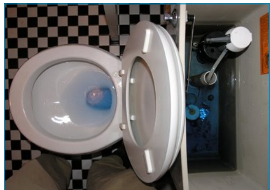
Toilet going through the food coloring test. This one has a leak!
